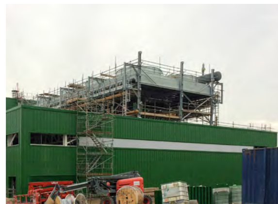
Holbrook Community Renewable Energy Centre roof mounted air cooled condensers
